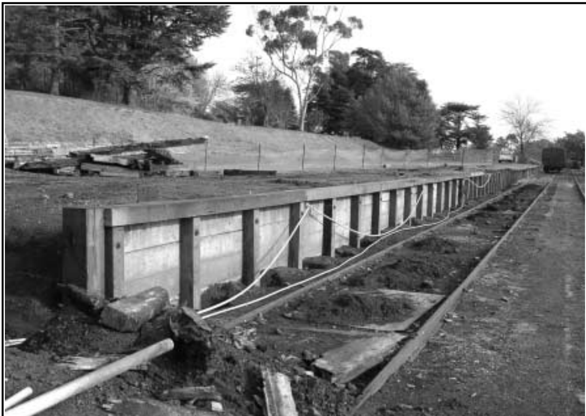
Contract work by Macleod Rail to renew the goods platform coping at Daylesford. May 2004. Photo: Barry Fell
