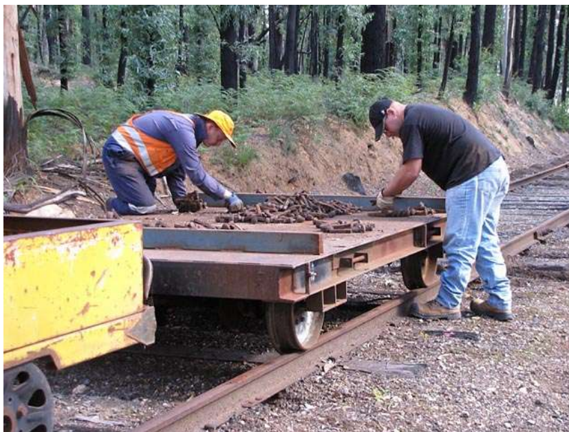
April 2010: Work goes ahead in the Fire Damaged section of the railway. Photo: Barry Fell
