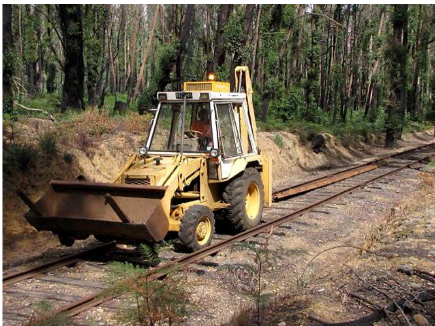
Dragging the new rail to location to replace that which buckled in the bushfire.
